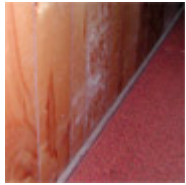
Mold on wooden paneling. (photo, Terry Brennan)
